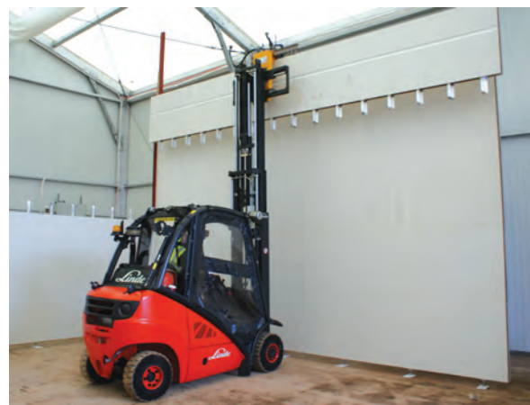
Panel courts (here ASB courts being installed at the University of Nottingham) allow versatile and quick construction
